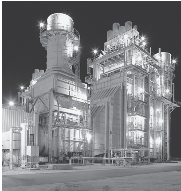
Natural gas-fired plants produce the majority of electricity in Texas.
