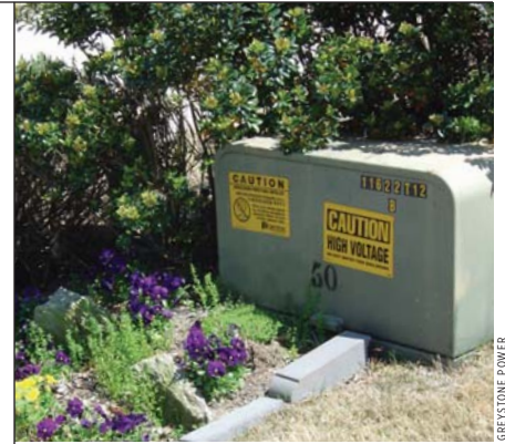
Never cover or block access to transformers.
